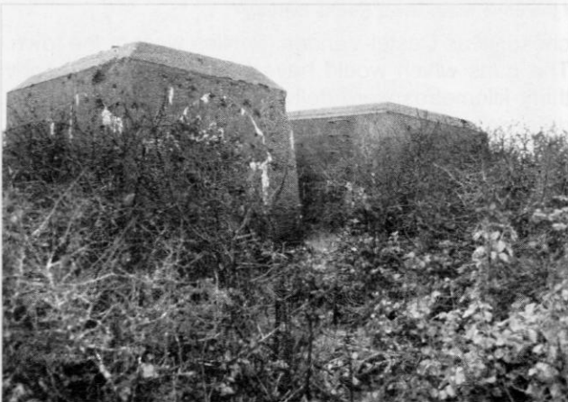
Support pillars for the Mammut radar array can on the roof of the Gouesneraie bunker
